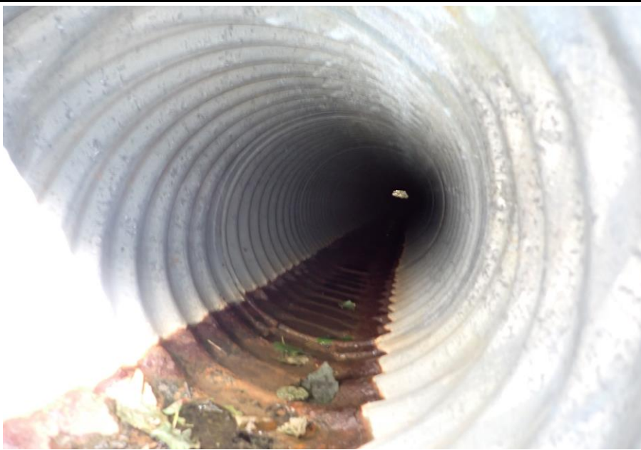
Bridge No. 1764 Br. Name Indian Creek Date 09/21/22 Inspector David McAdoo / Javier De Leon Frame 27 Looking Through FE US Culvert File P9210422.jpg
