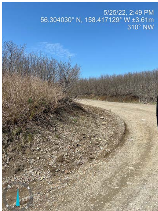
Washed Out Ditching Around Bend 2 of 2
