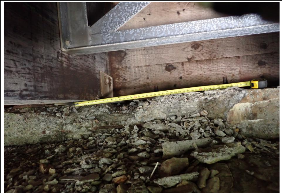
Bridge No. 1764 Br. Name Indian Creek Date 09/21/22 Inspector David McAdoo / Javier De Leon Frame 24 FE Abutment Cap Spall File P9210431.jpg
