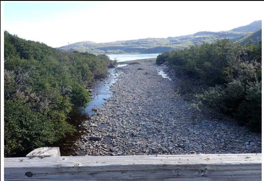
Bridge No. 1764 Br. Name Indian Creek Date 09/21/22 Inspector David McAdoo / Javier De Leon Frame 4 Looking DS File P9210409.jpg
