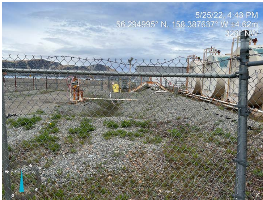
Pump Station 2 of 2
