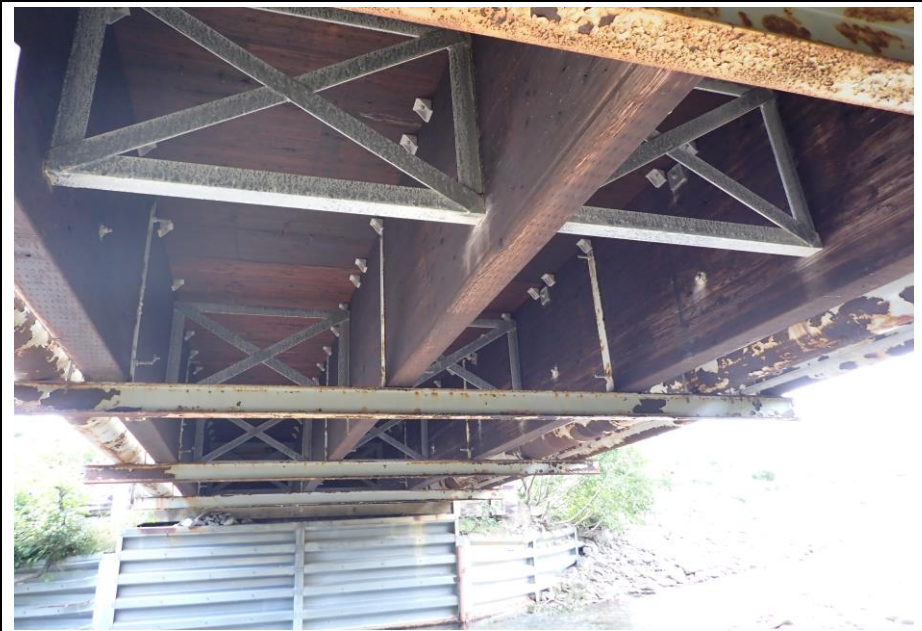
Bridge No. 1764 Br. Name Indian Creek Date 09/21/22 Inspector David McAdoo / Javier De Leon Frame 16 Deck Underside, Typ. File P9210429.jpg
