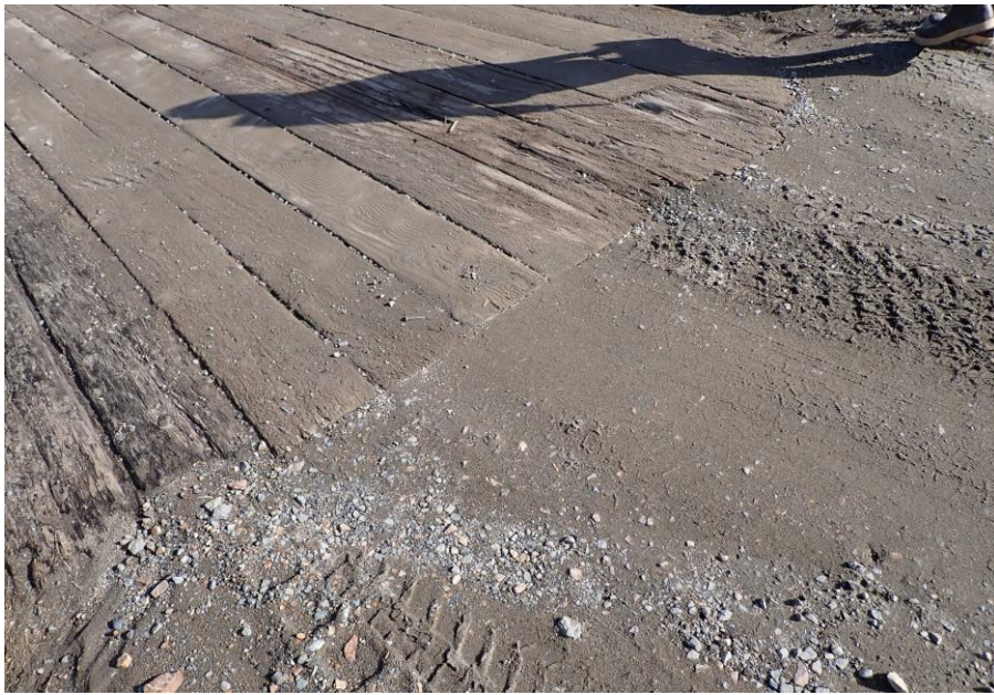
Bridge No. 1764 Br. Name Indian Creek Date 09/21/22 Inspector David McAdoo / Javier De Leon Frame 9 NE Joint File P9210407.jpg
