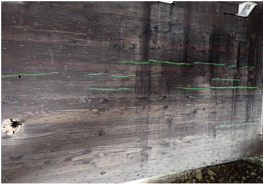
Bridge No. 1764 Br. Name Indian Creek Date 09/21/22 Inspector David McAdoo / Javier De Leon Frame 25 Girder 1 FE DS Face Splits File P9210432.jpg
