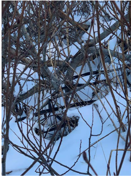
9 - Exposed Electric Service Line
