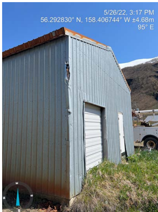
Damaged Siding 1 of 2
