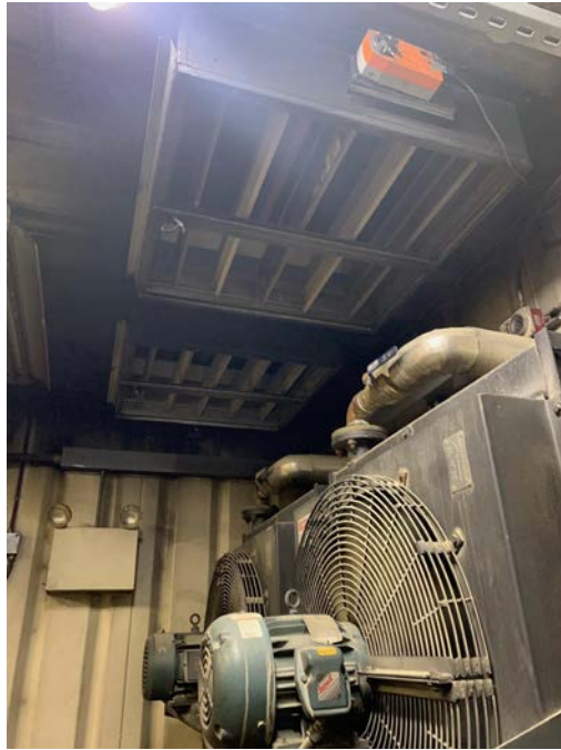
19 - Radiators and Fans
