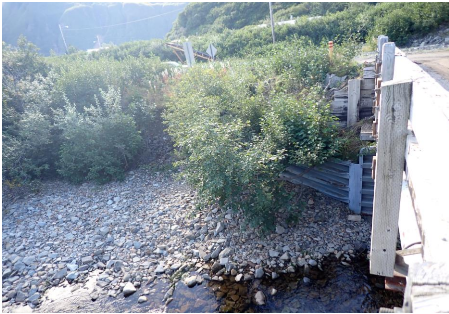
Bridge No. 1764 Br. Name Indian Creek Date 09/21/22 Inspector NE DS David McAdoo / Javier De Leon Frame 5 File P9210410.jpg
