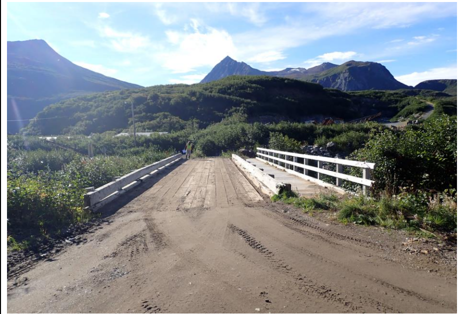
Bridge No. 1764 Br. Name Indian Creek Date 09/21/22 Inspector David McAdoo / Javier De Leon Frame 2 Back at Bridge File P9210418.jpg
