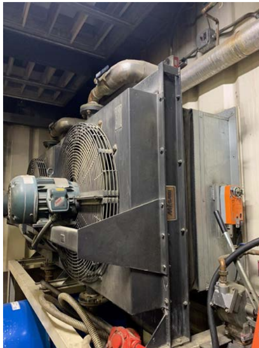
18 - Radiators and Fans
