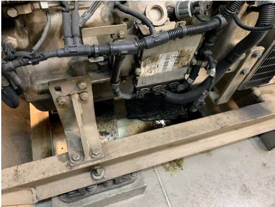
37 - #3 Engine Oil Leak
