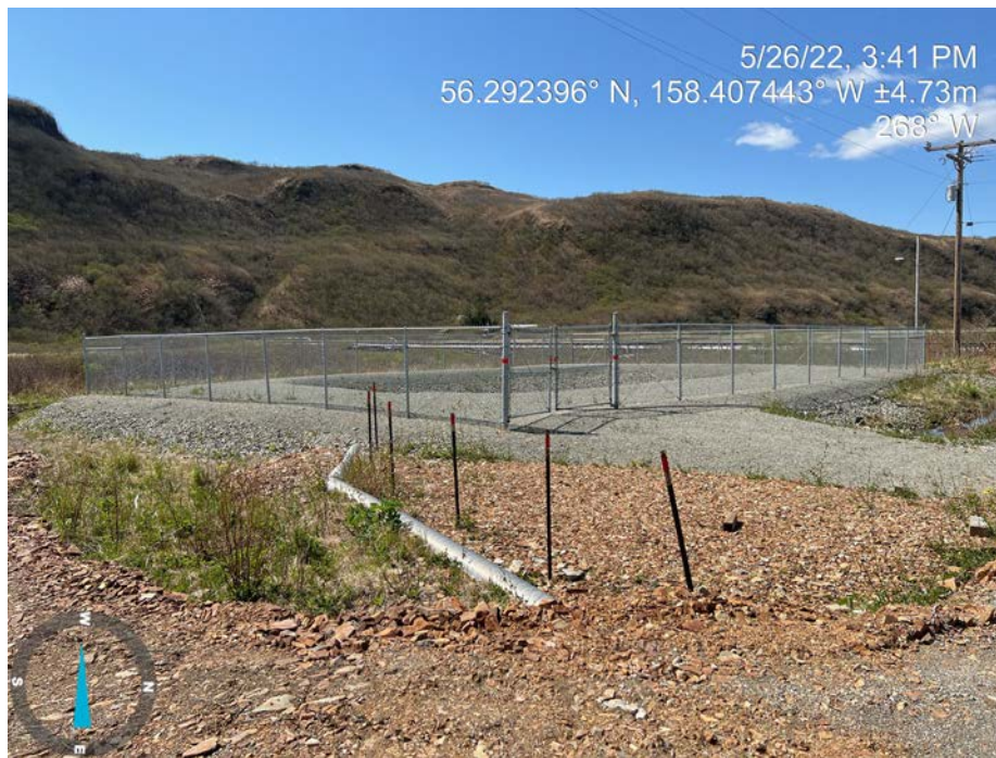
Pipe from Water Treatment Plant
