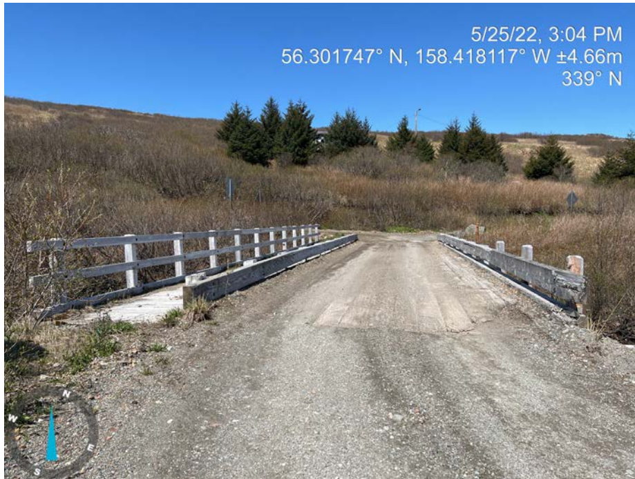
Damaged Decking & Rub Rails
