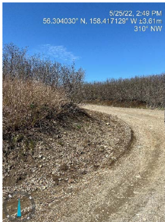
Washed Out Ditching Around Bend
