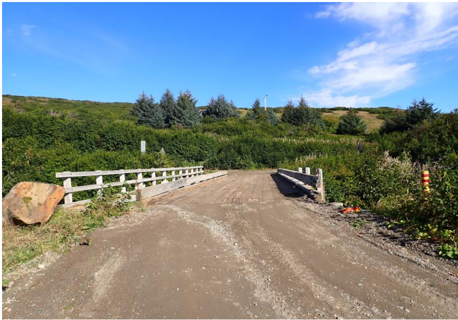
Bridge No. 1764 Br. Name Indian Creek Date 09/21/22 Inspector David McAdoo / Javier De Leon Frame 1 Ahead at Bridge File P9210406.jpg
