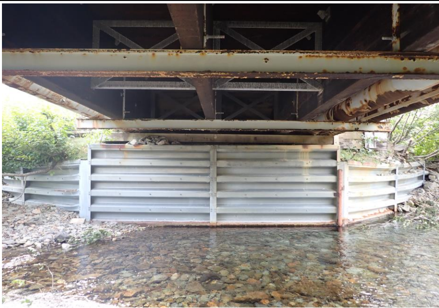
Bridge No. 1764 Br. Name Indian Creek Date 09/21/22 Inspector David McAdoo / Javier De Leon Frame 11 NE Abutment File P9210434.jpg
