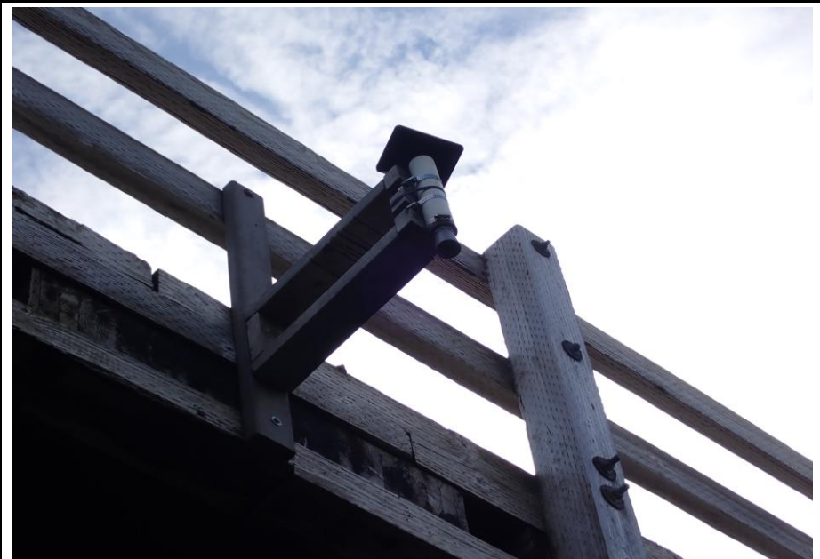
Bridge No. 1764 Br. Name Indian Creek Date 09/21/22 Inspector David McAdoo / Javier De Leon Frame 32 FE US Stream Gauge File P9210427.jpg
