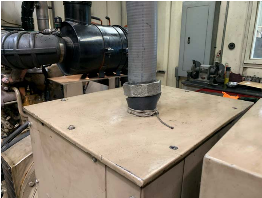
28 - #3 Generator Chafed Wire Temporary Fix
