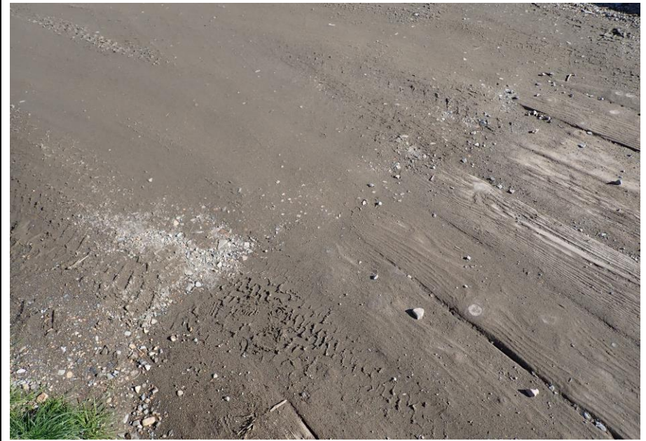
Bridge No. 1764 Br. Name Indian Creek Date 09/21/22 Inspector David McAdoo / Javier De Leon Frame 10 FE Joint File P9210417.jpg
