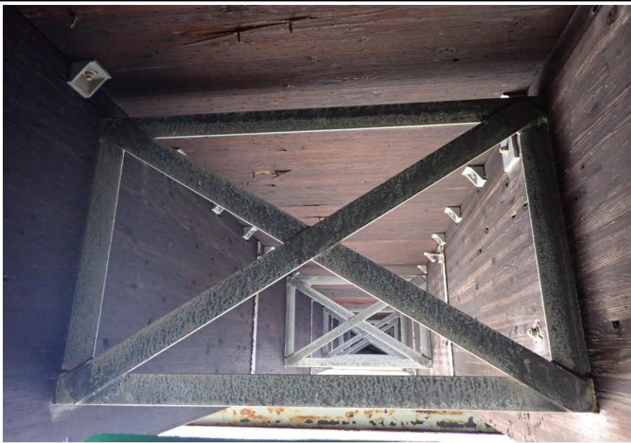
Bridge No. 1764 Br. Name Indian Creek Date 09/21/22 Inspector David McAdoo / Javier De Leon Frame 15 Crossframe, Typ. File P9210426.jpg
