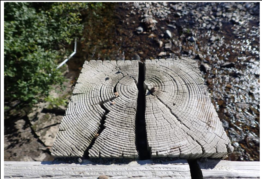
Bridge No. 1764 Br. Name Indian Creek Date 09/21/22 Inspector David McAdoo / Javier De Leon Frame 20 Rail Post, Typ. File P9210415.jpg
