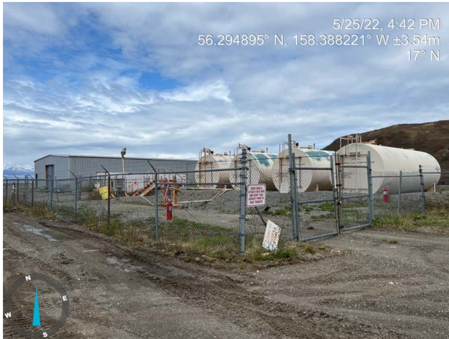
Diesel Fuel Tanks
