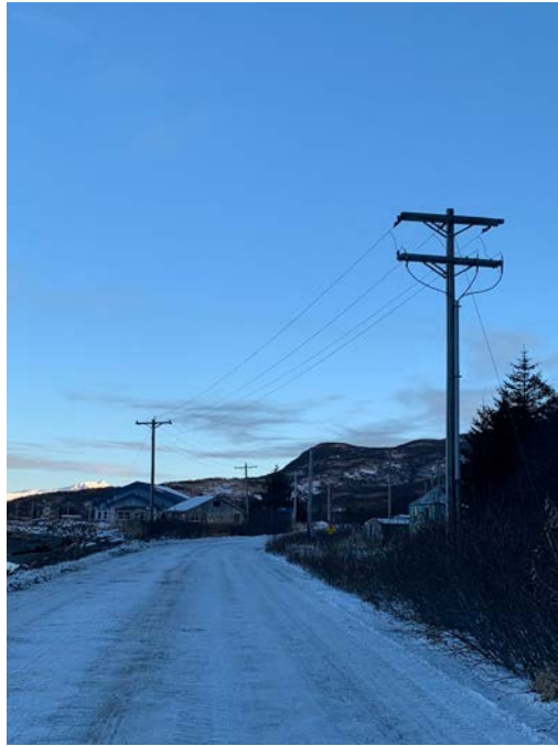
21 - Start of East Side Electric Poles
