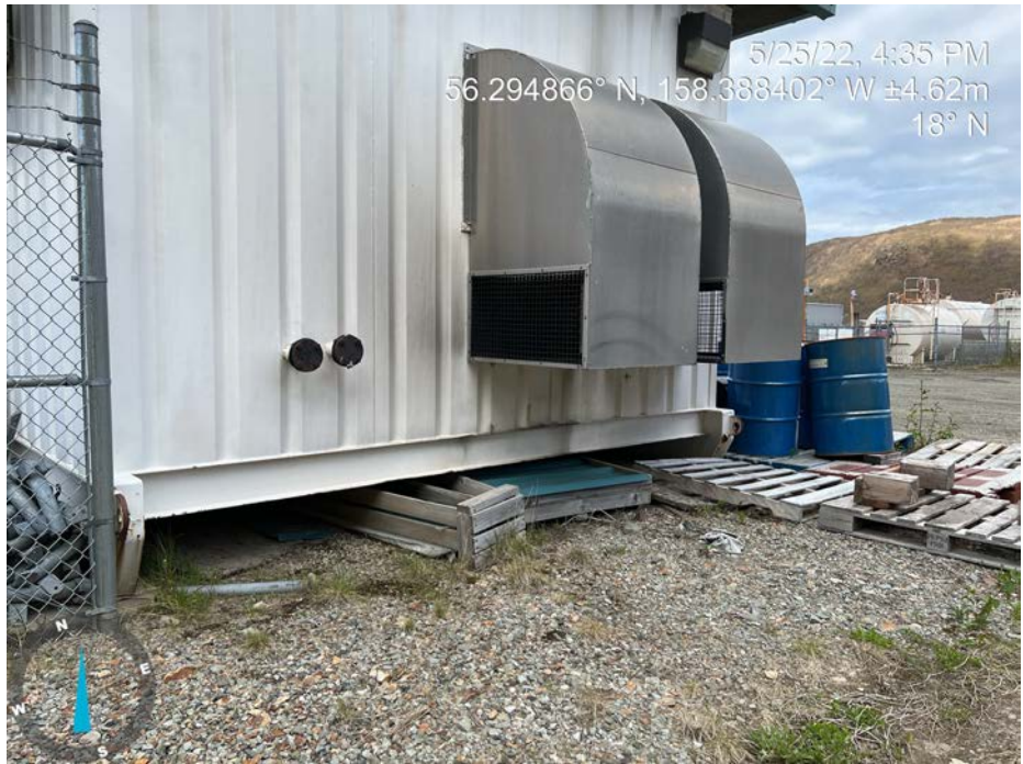
Metal Skid Foundation
