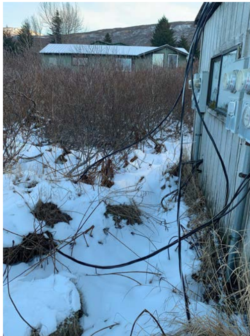
8 - Exposed Electric Service Line
