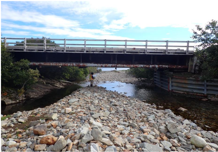
Bridge No. 1764 Br. Name Indian Creek Date 09/21/22 Inspector David McAdoo / Javier De Leon Frame 17 Elevation from US File P9210433.jpg
