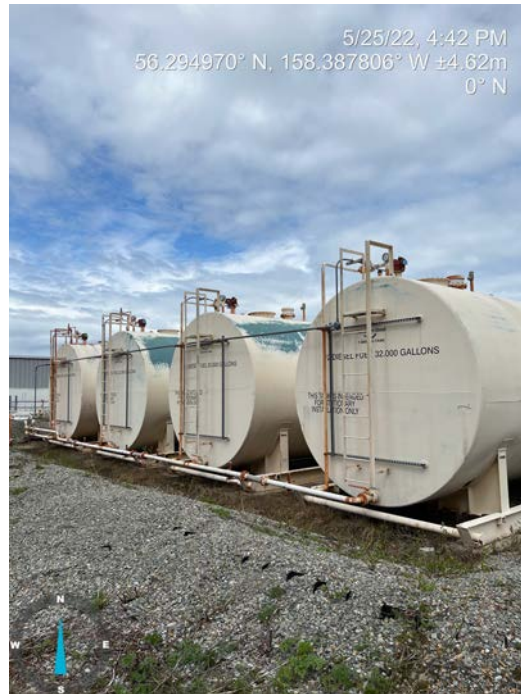
Metal Skid & Fuel Rails
