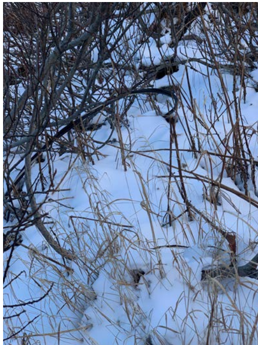
10 - Exposed Electric Service Line
