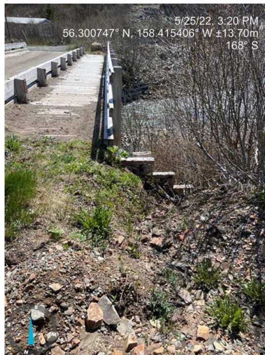
Erosion at South Abutment Wood Wing Wall
