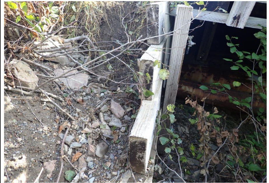
Bridge No. 1764 Br. Name Indian Creek Date 09/21/22 Inspector David McAdoo / Javier De Leon Frame 22 FE US Backwall Separation File P9210423.jpg
