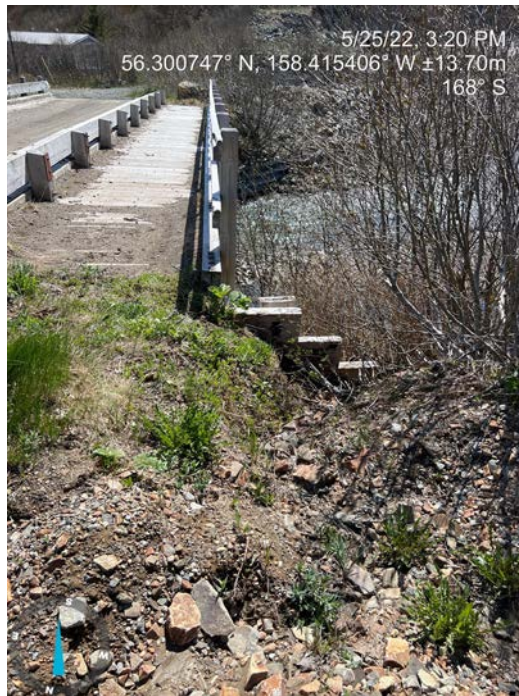
Erosion at South Abutment Wood Wing Wall
