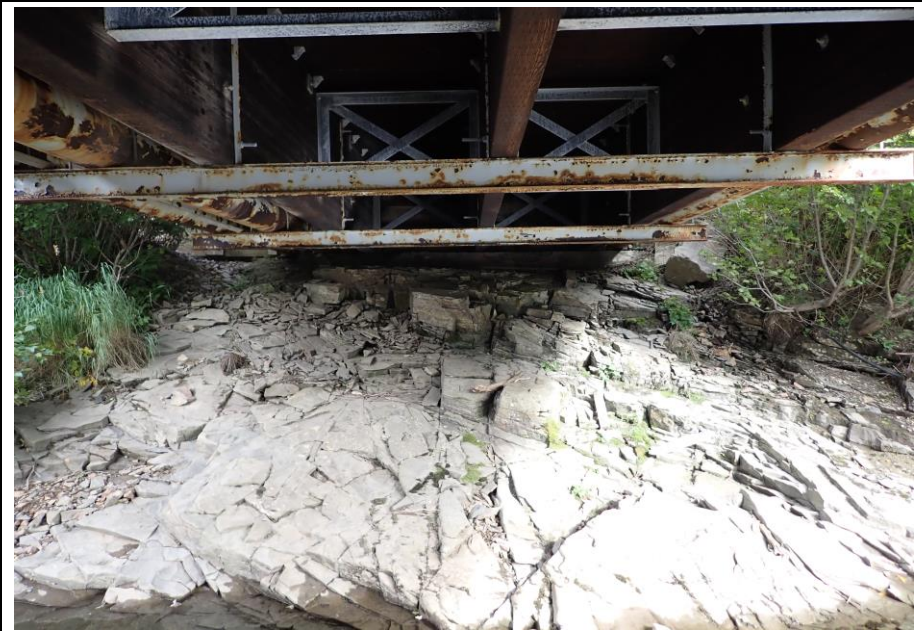
Bridge No. 1764 Br. Name Indian Creek Date 09/21/22 Inspector David McAdoo / Javier De Leon Frame 12 FE Abutment File P9210435.jpg
