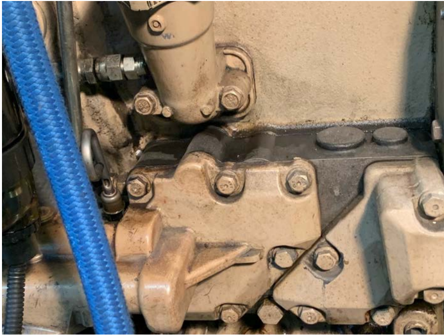
35 - #3 Engine Oil Leak
