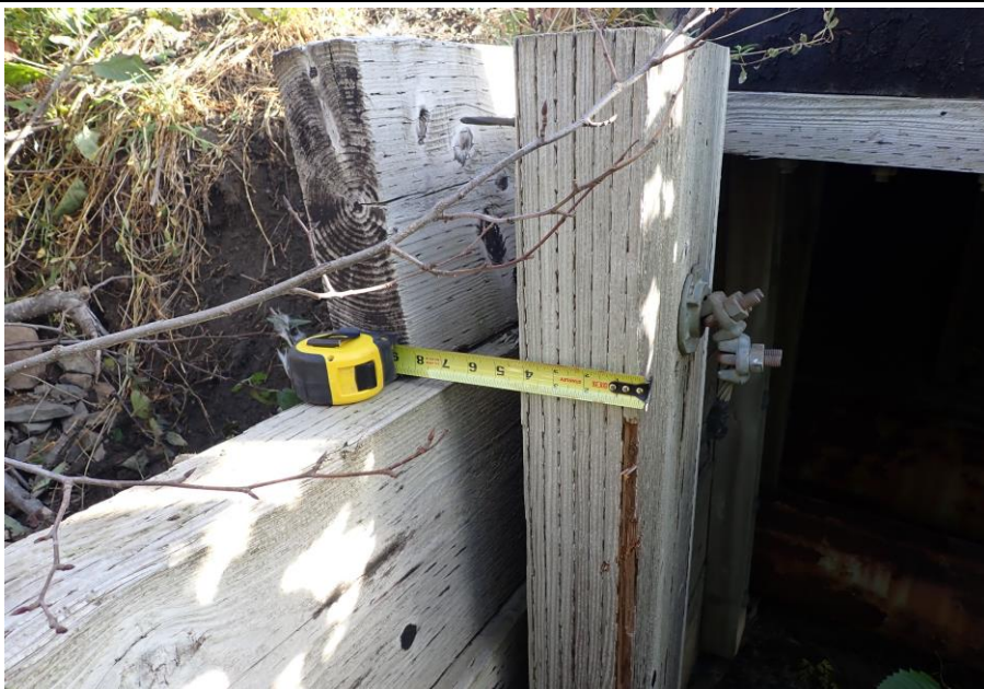
Bridge No. 1764 Br. Name Indian Creek Date 09/21/22 Inspector David McAdoo / Javier De Leon Frame 23 FE US Backwall Separation File P9210424.jpg
