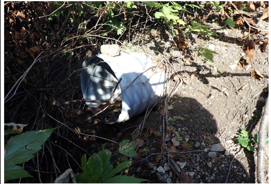
Bridge No. 1764 Br. Name Indian Creek Date 09/21/22 Inspector David McAdoo / Javier De Leon Frame 26 FE US Culvert Outlet File P9210421.jpg
