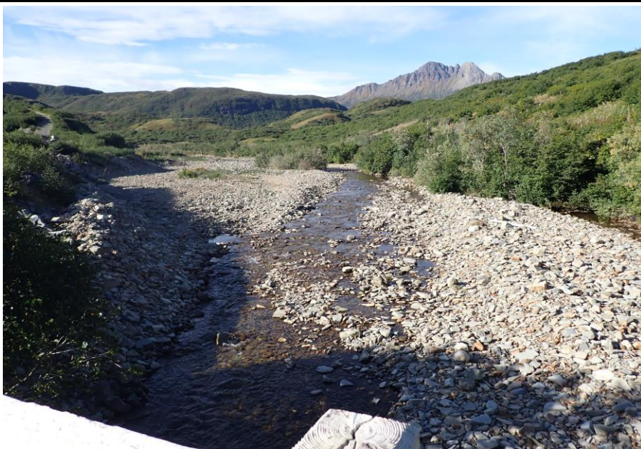
Bridge No. 1764 Br. Name Indian Creek Date 09/21/22 Inspector David McAdoo / Javier De Leon Frame 3 Looking US File P9210412.jpg
