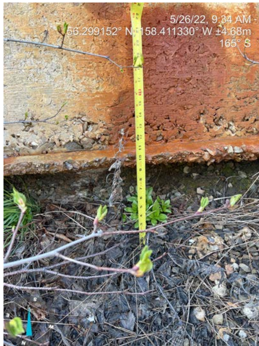
Foundation Pitting & Lack of Fill 1 of 2
