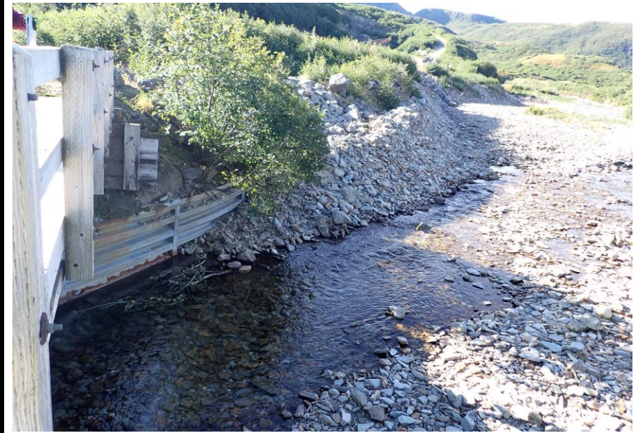
Bridge No. 1764 Br. Name Indian Creek Date 09/21/22 Inspector NE US David McAdoo / Javier De Leon Frame 6 File P9210414.jpg
