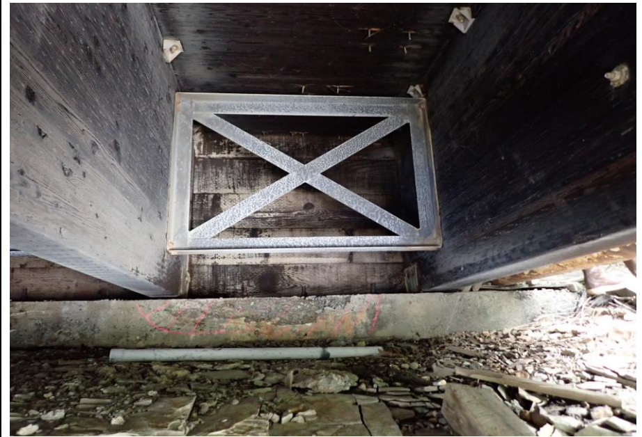
Bridge No. 1764 Br. Name Indian Creek Date 09/21/22 Inspector David McAdoo / Javier De Leon Frame 14 FE Abutment Bay 2, Typ. File P9210428.jpg
