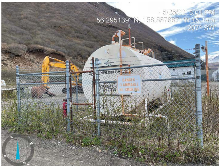
Gasoline Fuel Tank 1 of 2
