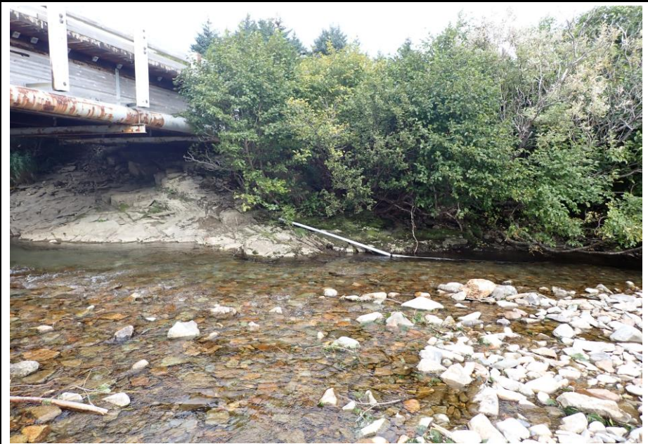
Bridge No. 1764 Br. Name Indian Creek Date 09/21/22 Inspector David McAdoo / Javier De Leon Frame 28 FE DS Unknown Utility File P9210438.jpg
