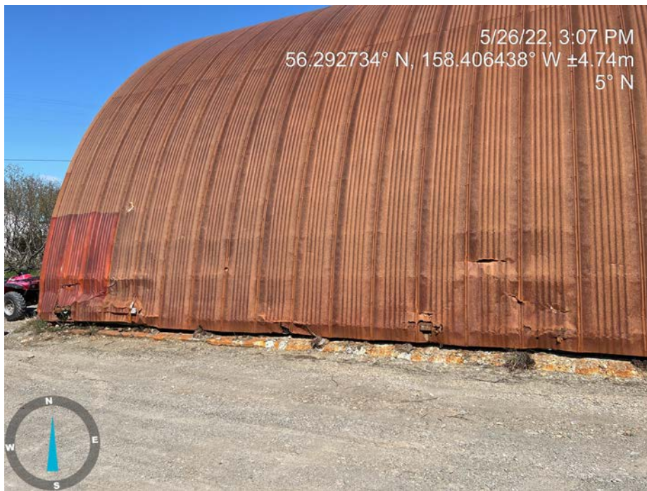
Damaged Exterior Dome 1 of 2
