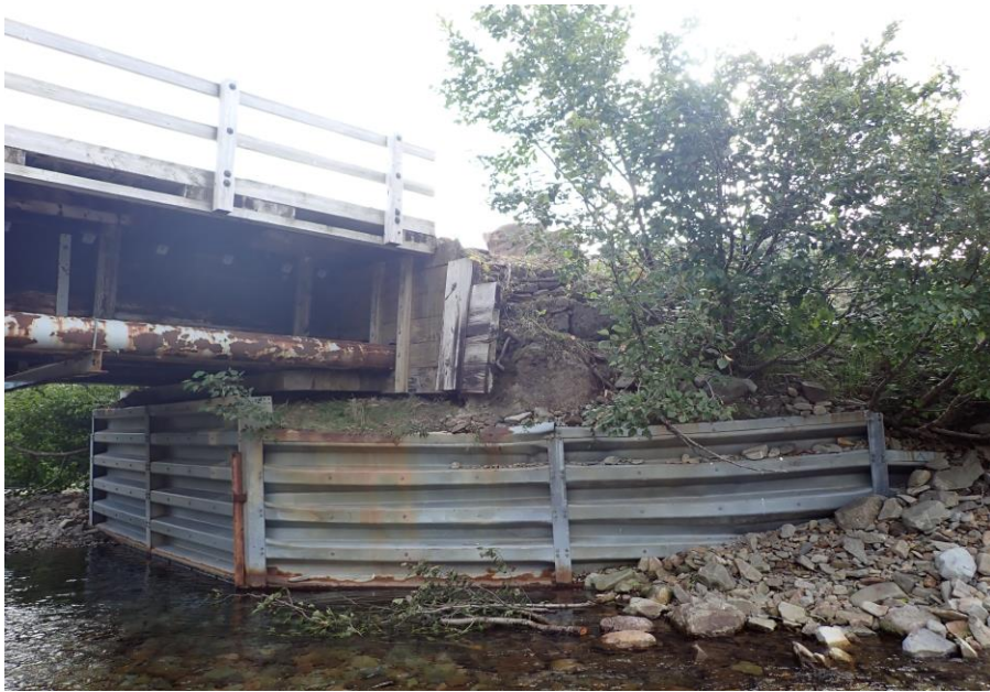
Bridge No. 1764 Br. Name Indian Creek Date 09/21/22 Inspector David McAdoo / Javier De Leon Frame 21 NE US Backwall Separation File P9210436.jpg
